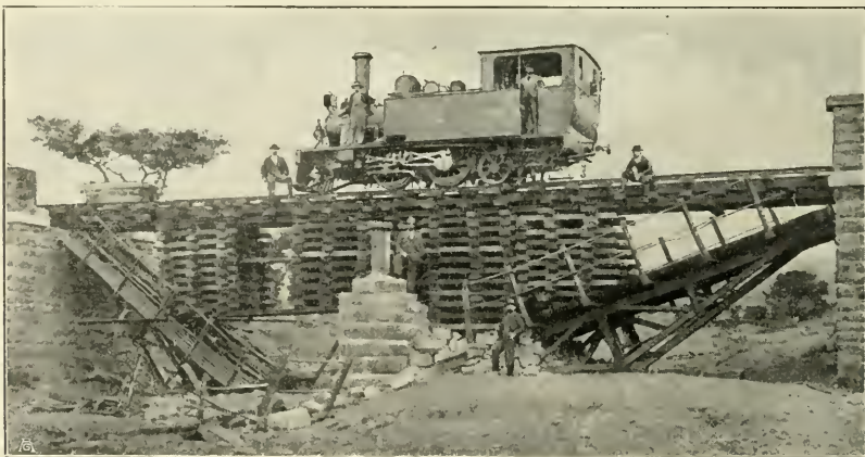
THE RAILWAY BRIDGE OVER THE SUNDAY RIVER (NATAL), REPAIRED BY THE TRANSVAALERS. The English repair bridges in the same manner, or else build a kind of bridge in the bed of the river. These are, of course, only make-shifts, and quite unable to resist the rapids, especially after the tropical rains, when the force of the current becomes exceedingly strong.
